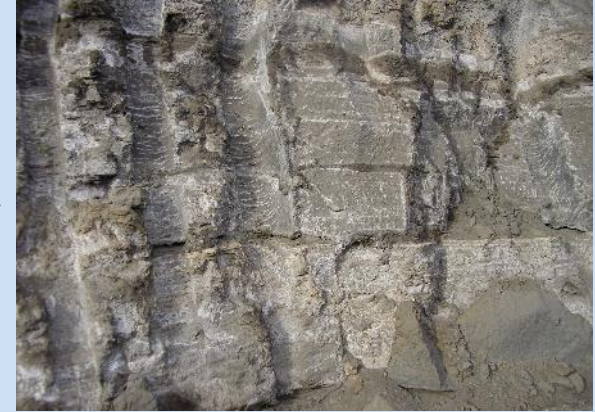
Desiccation and cementation
