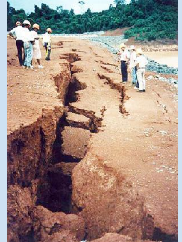
Engineering defects – internal erosion
